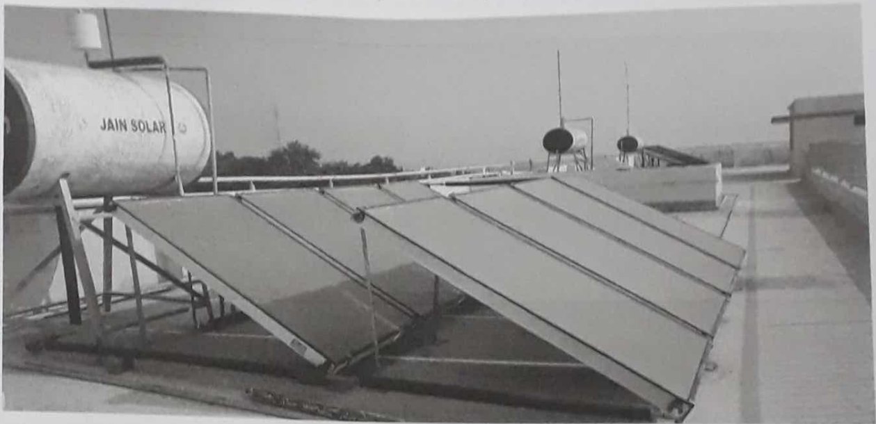
Solar water geysers at Girls Hostel
